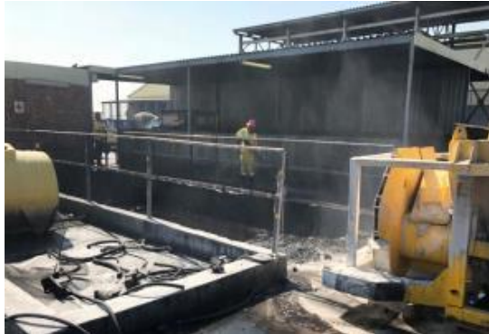
Photograph 7-6: Sump Located at Wash Bay
