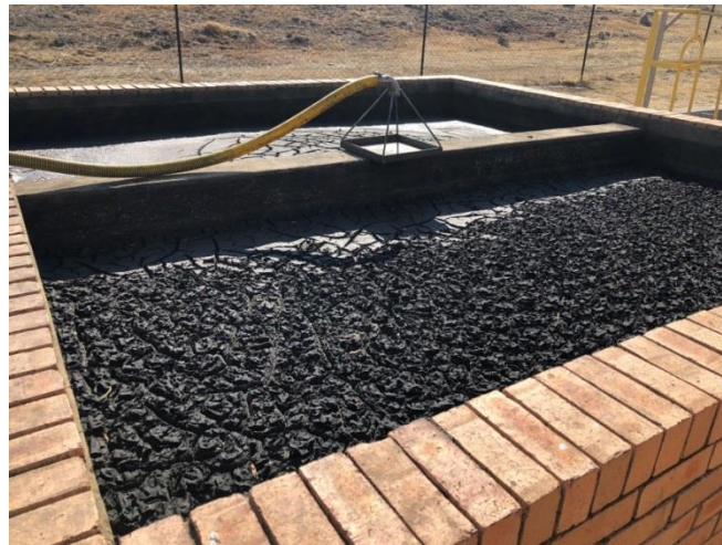
Figure 5-19: STP - Sludge drying beds
