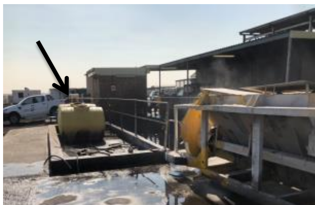
Figure 5-15: Oil skimmers located at wash bay
