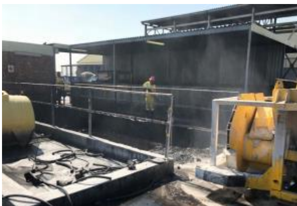
Figure 5-14: Sump located at wash bay
