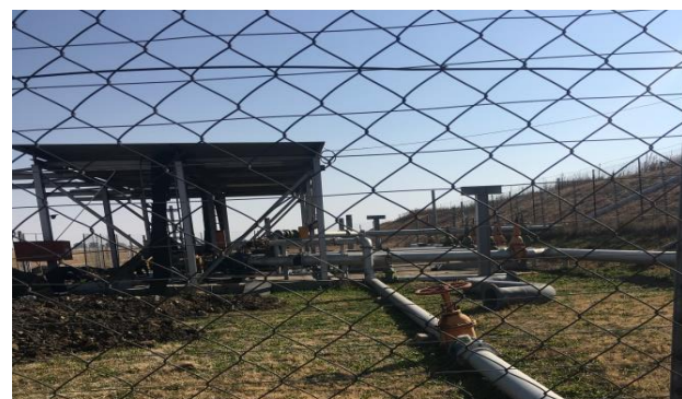
Figure 5-12: Existing pump station
