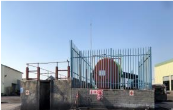
Figure 5-20: Fuel and oil storage area
