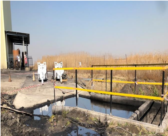
Figure 5-16: Sump located at workshop and oil storage area
