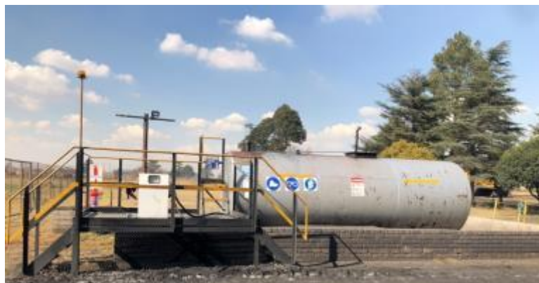
Figure 5-22: Diesel Storage Facility at 3 Shaft
