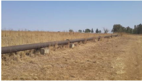
Figure 11-35: Detail of existing ash pipeline. Note the low impact on the landscape
