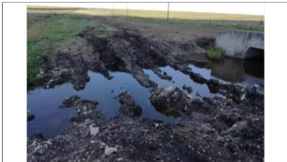
Photograph 5-4: Altered stream channel geometry and silted river at a crossing
