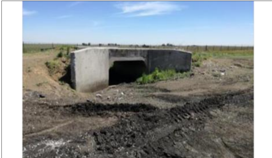
Photograph 5-3: Altered stream channel geometry and silted river at a crossing
