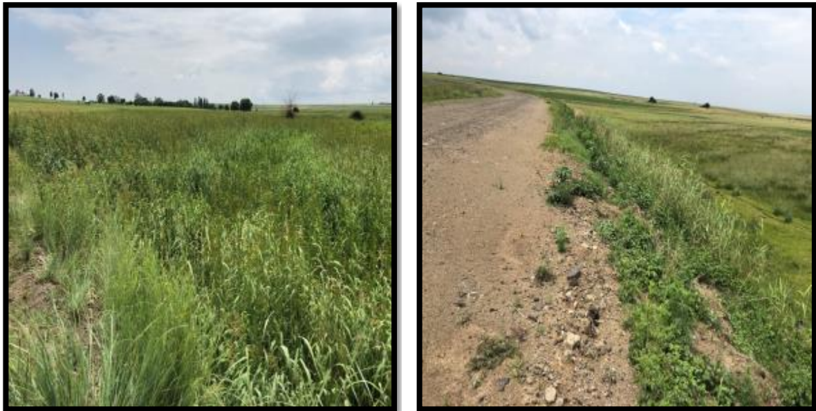
Figure 5-19: Access road to Twistdraai East Shaft (Between Mynpad Road and the Twistdraai East Shaft) after tar removal
