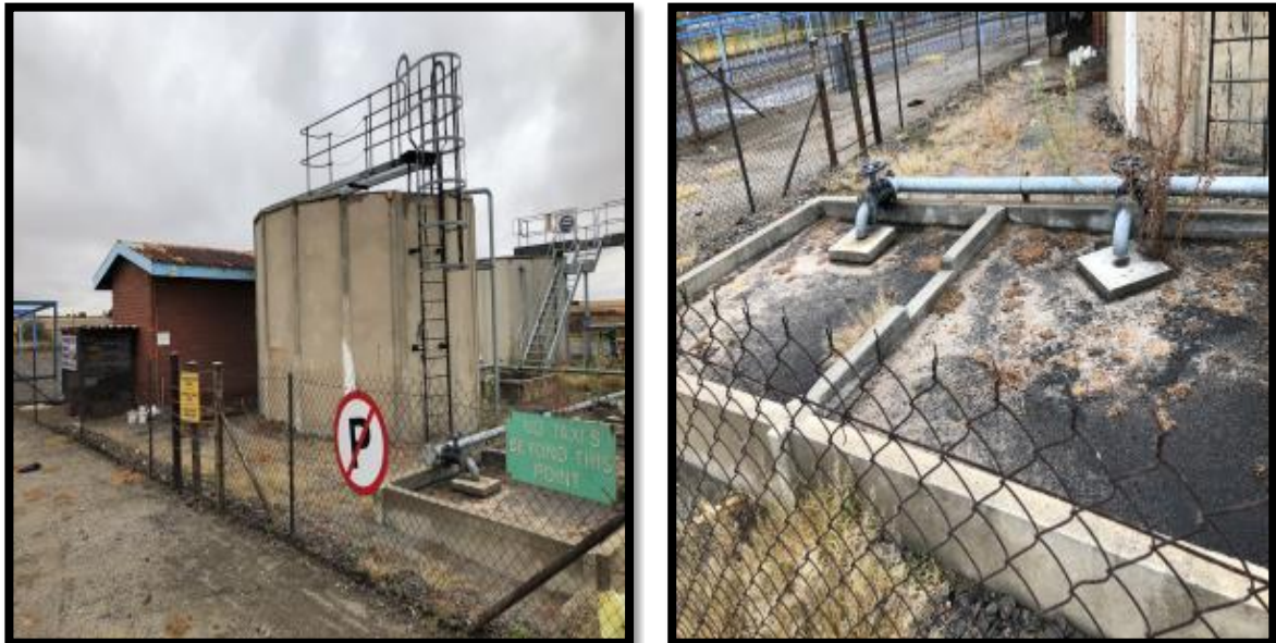
Figure 5-10: Sewage Treatment Plant prior to decommissioning
