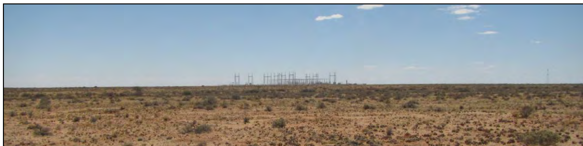
Figure 3: View towards the northeast of the Eskom Nieuwehoop Substation currently under construction at the northern end of the electrical corridor.
