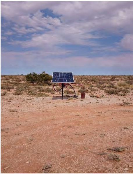
BH7 – solar pump borehole
