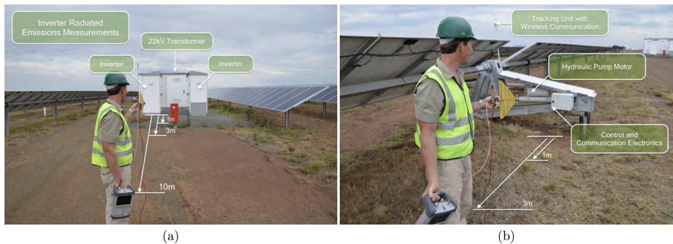
Figure 15: Radiated measurements of (a) Inverter and Transformer units and (b) Tracking Cabinet.
