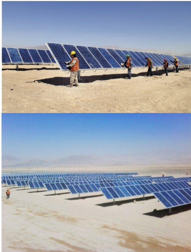
Figure 1: Solar PV facility (Courtesy of Kabi Solar)
