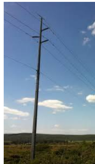
Plate 3, Eskom 132kV Monopole.
