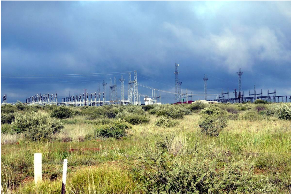
Plate 1, Existing Mookodi 400/132kV Substation.
