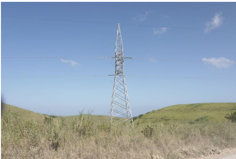
Plate 2, Eskom 132kV Lattice Tower 25-28m high. 132kV structures will be slightly higher than existing and will follow the existing power line servitude.
