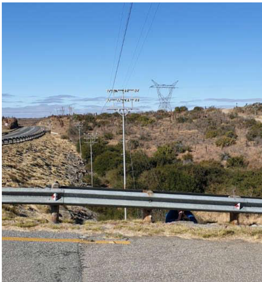
Figure 3-7: Overhead lines at Access Point 2
