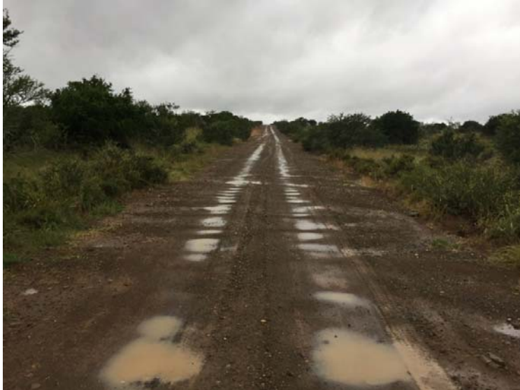
Figure 3 – Condition of District Road DR02462
