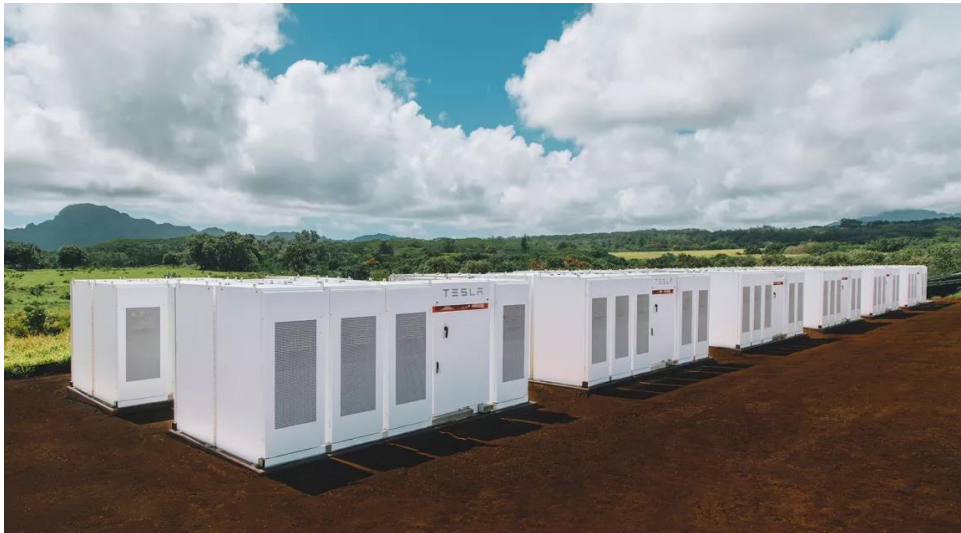
Figure 3.5: Example of battery storage units installed by Tesla (Source: fastcompany.com)
