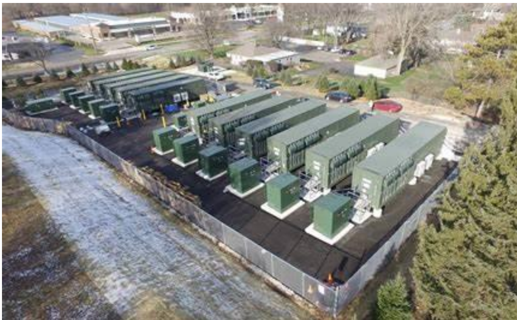
Plate 1 - Typical Battery Energy Storage System
