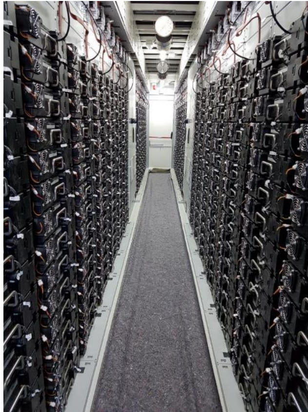
Figure 4.7: Li-Ion BESS internal design and implementation of a container used within a BESS. The image shows a series of sealed battery cell packs within a containerised module (Source: Enel Green Power).
