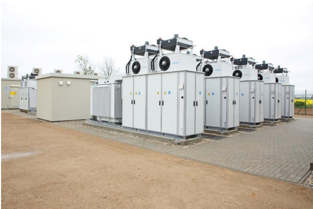
Figure 4.6: Li-Ion BESS containerised modules located within the BESS enclosure footprint (Source: Enel Green Power).
