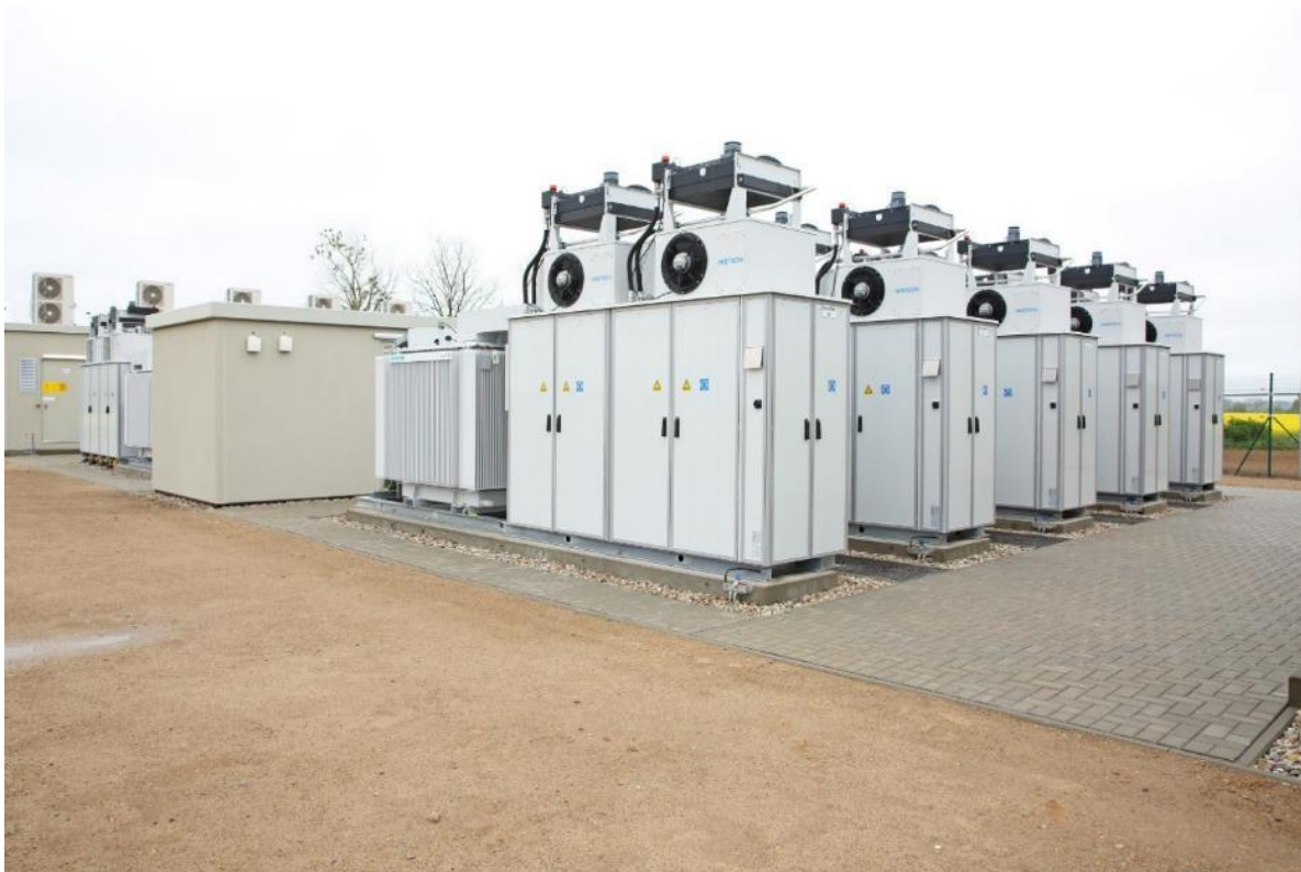
Figure 4.6: Li-Ion BESS containerised modules located within the BESS enclosure footprint (Source: Enel Green Power).
