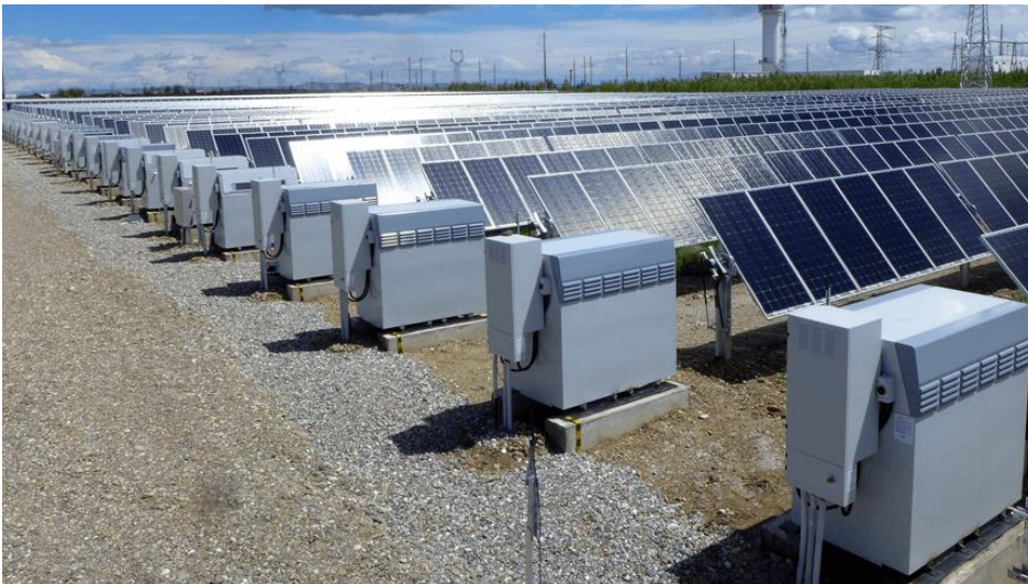
Figure 7.10 Example of battery storage units integrated as part of PV array (Source: nexttracker.com)
