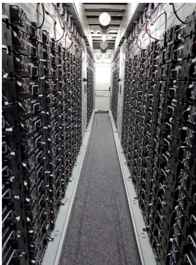
Figure 4.7: Li-Ion BESS internal design and implementation of a container used within a BESS. The image shows a series of sealed battery cell packs within a containerised module (Source: Enel Green Power).
