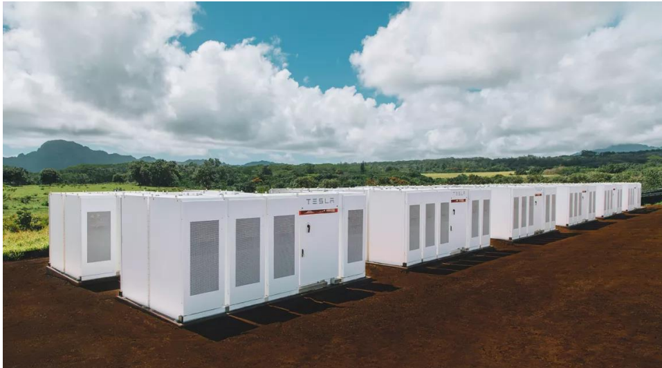
Figure 0.2: Example of battery storage units installed by Tesla (Source: fastcompany.com)
