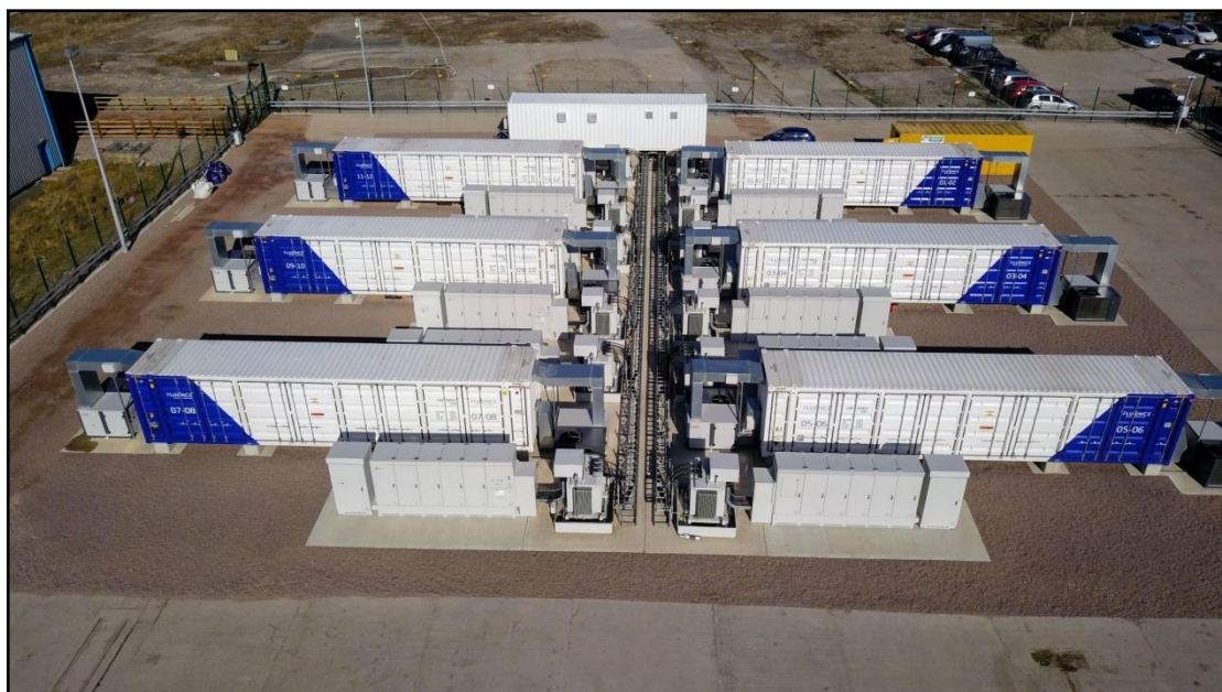
Figure 4: Aerial view of a BESS facility (Photo: Power Engineering International).
