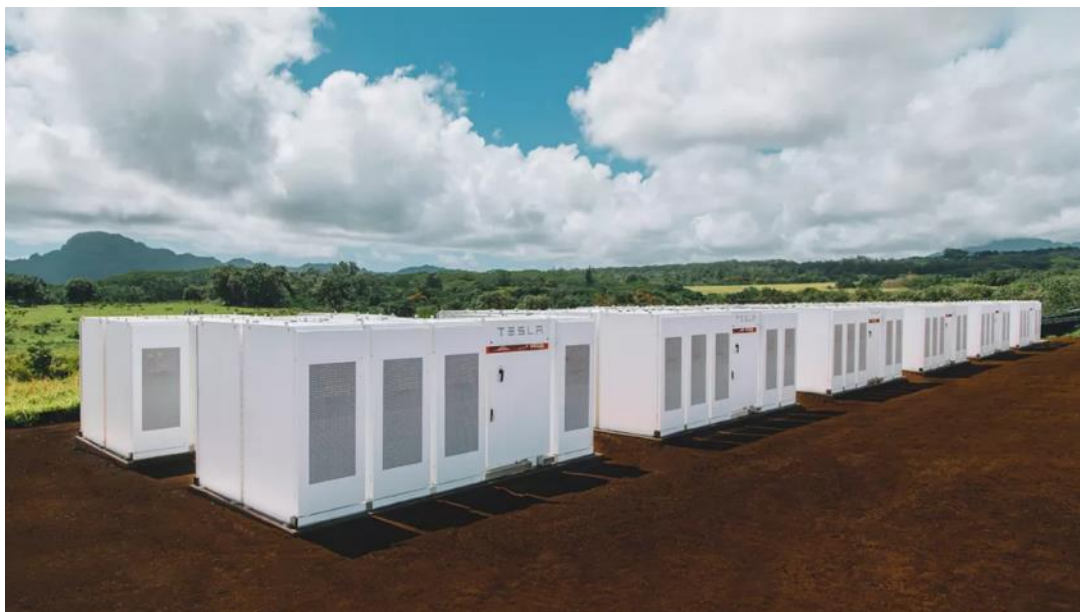
Figure 4.8: Illustration of battery storage units installed by Tesla (Source: fastcompany.com).
