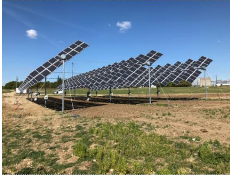
Figure 11: Photo of the EDF agrivoltaic demonstrator located in Ecuellas (France)
