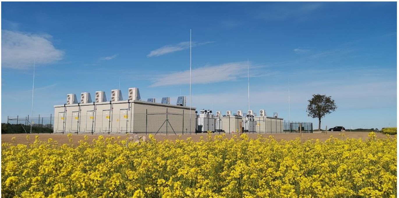
Figure 4.5: Li-Ion BESS implementation for a Renewable Energy facility (Source: Enel Green Power).
