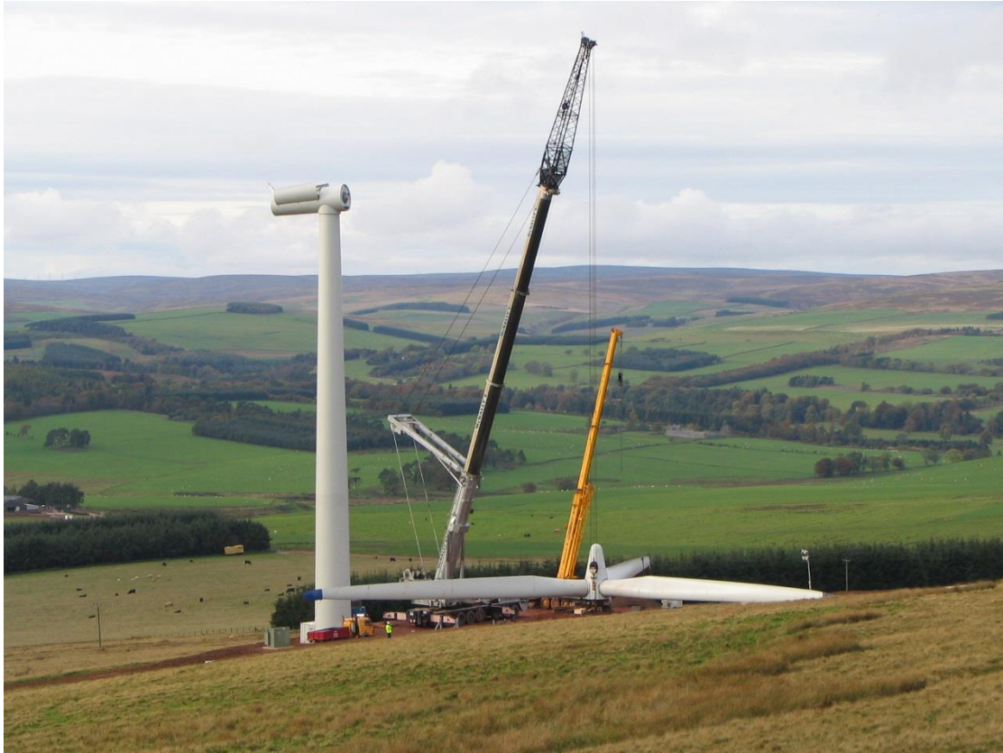
Figure 4.3: Example of a tower on which the rotor is mounted
