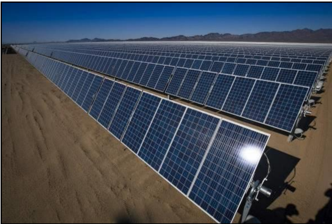
Photograph 1.1: Typical PV SEF facility
