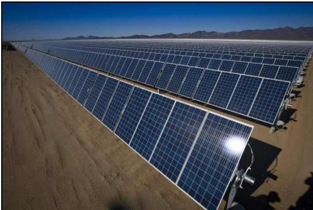
Photograph 1.1: Typical PV SEF facility
