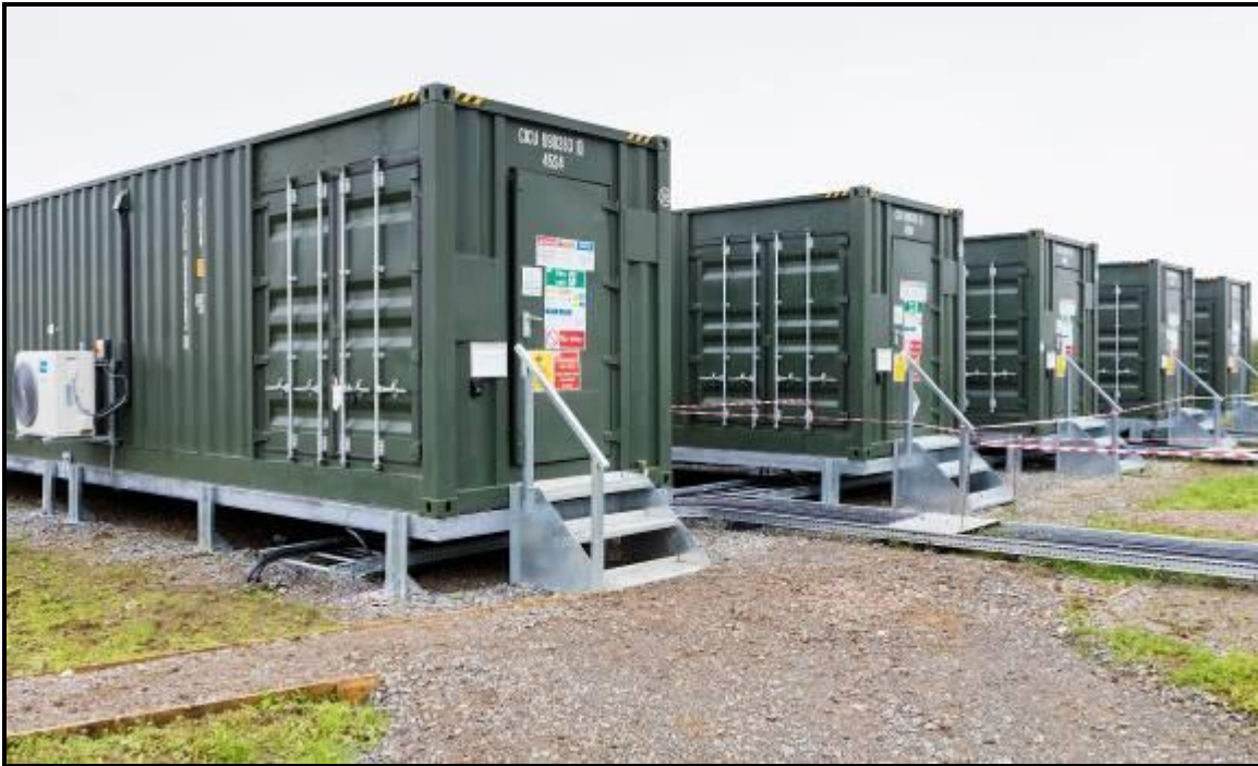
Photograph 1.2: Example of BESS located in storage containers
