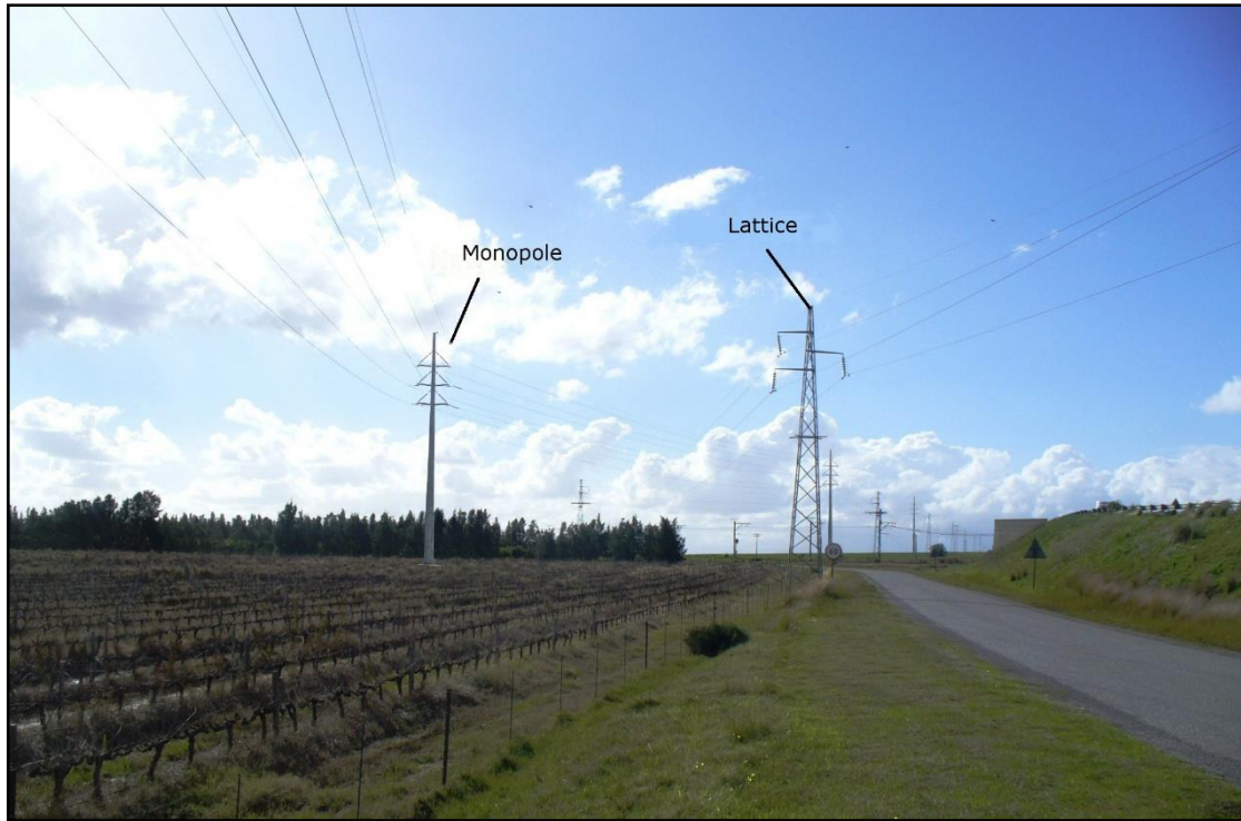
Figure 3: Typical 132kV power line structures.
