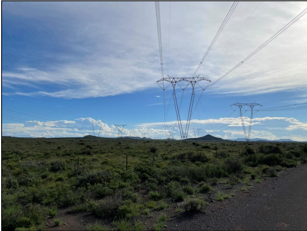
Figure 6: Existing power lines crossing the Hutchinson secondary road (looking to the south-west).
