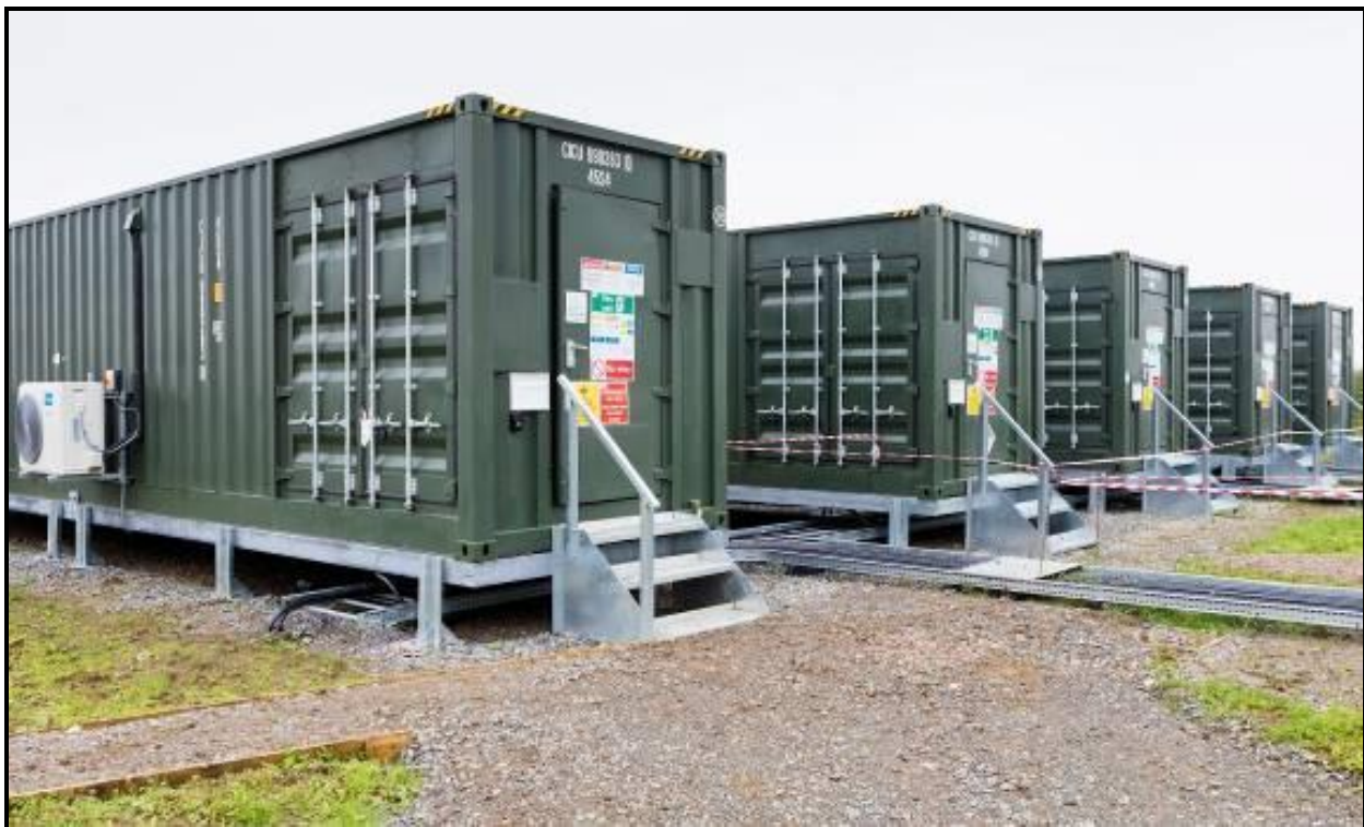
Photograph 1.1: Example of BESS located in storage containers
