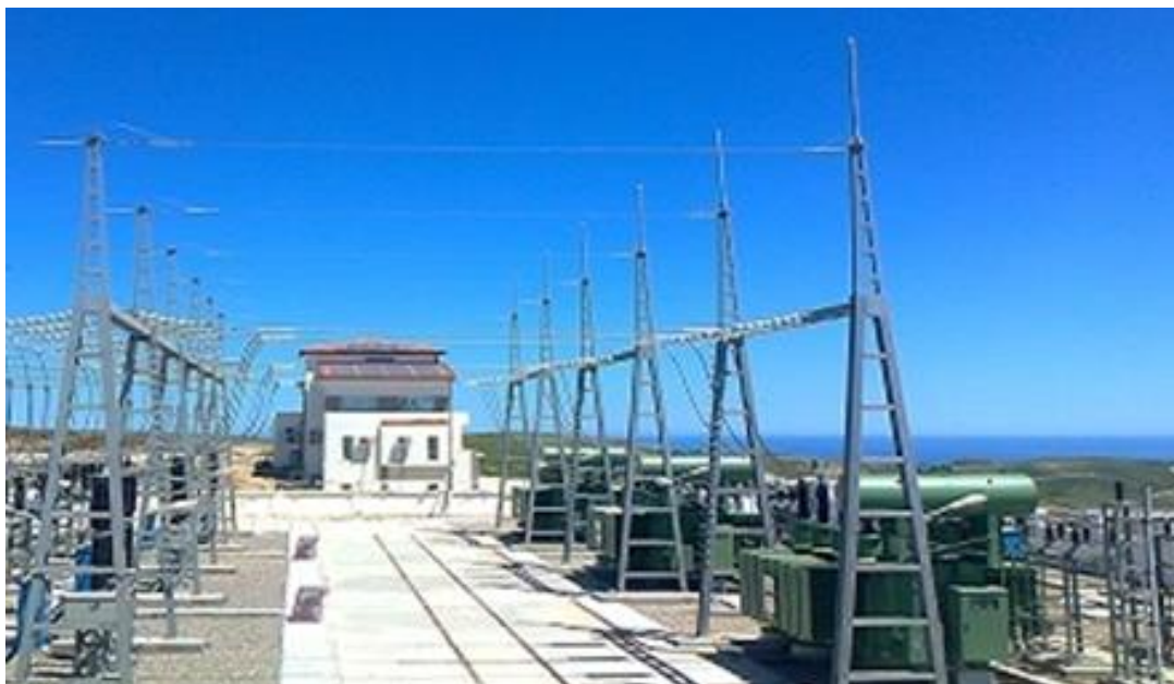
PLATE 2, BUS BARS (TALL STRUCTURES CENTRE AND LEFT OF IMAGE) ARE THE HIGHEST SUBSTATION ELEMENTS IN PICTURE.
