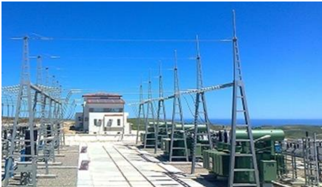
PLATE 2, BUS BARS (TALL STRUCTURES TO CENTRE AND LEFT OF IMAGE) ARE THE HIGHEST SUBSTATION ELEMENTS IN PICTURE.
