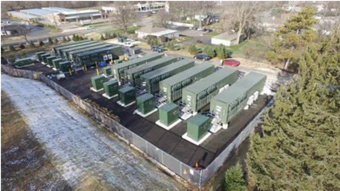
PLATE 3 - TYPICAL BATTERY ENERGY STORAGE SYSTEM
