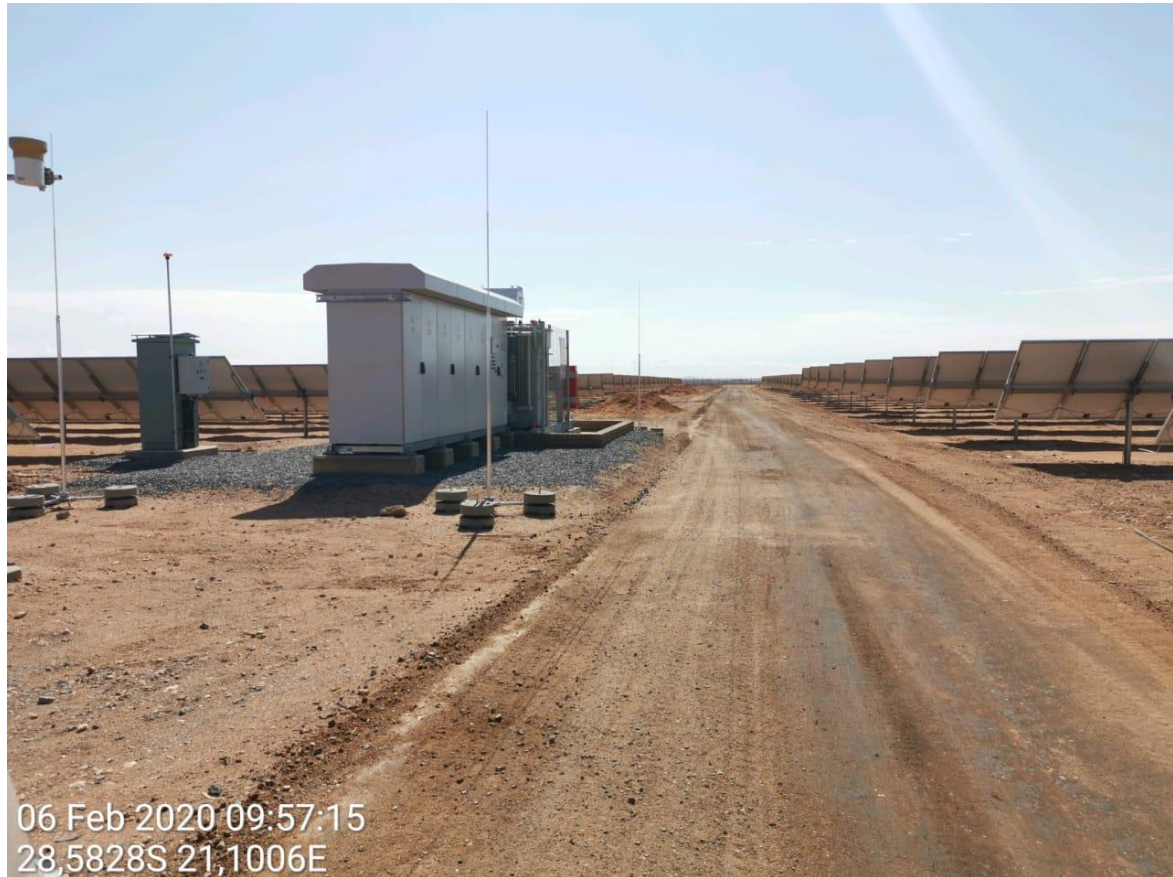
Plate 1, VIEW OF TRACKING ARRAY WITH CENTRALISED INVERTER STATION IN THE FOREGROUND
