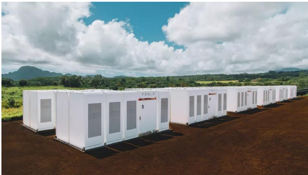
Figure 2.11: Illustration of battery storage units installed by Tesla (Source: fastcompany.com).
