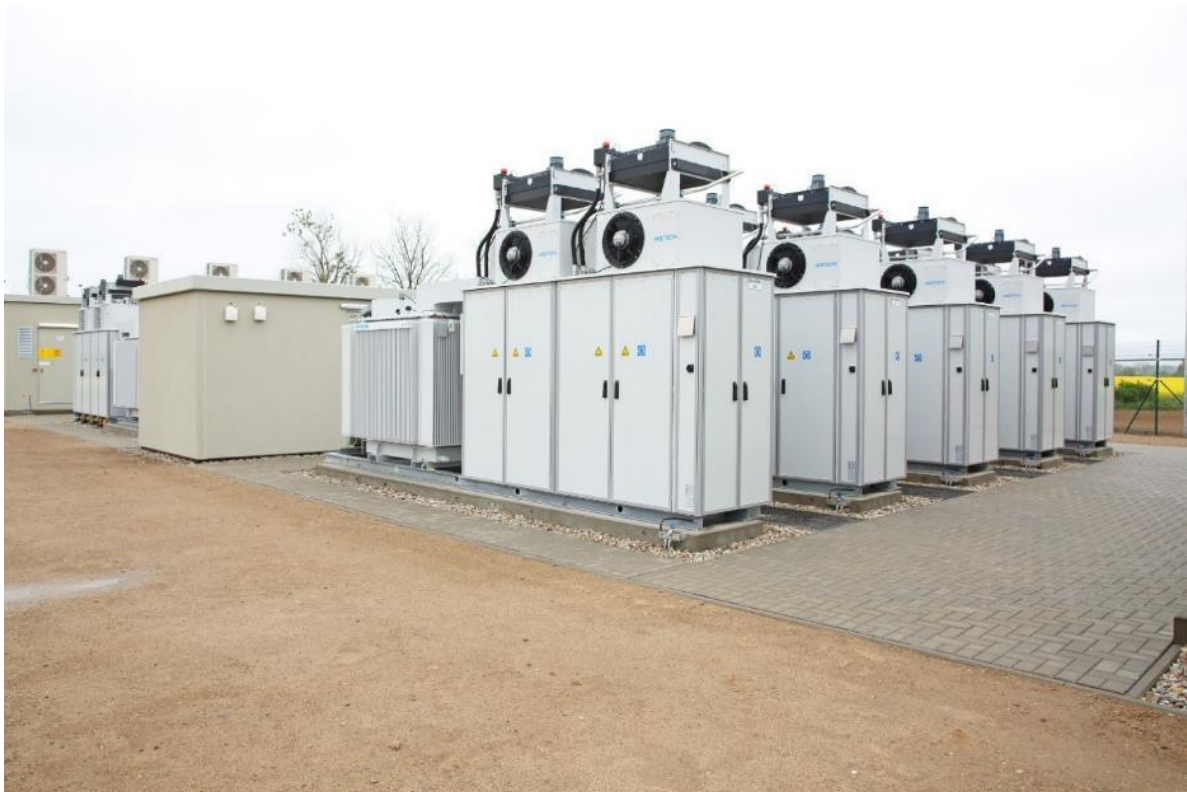
Figure 2.9: Li-Ion BESS containerised modules located within the BESS enclosure footprint (Source: Enel Green Power).
