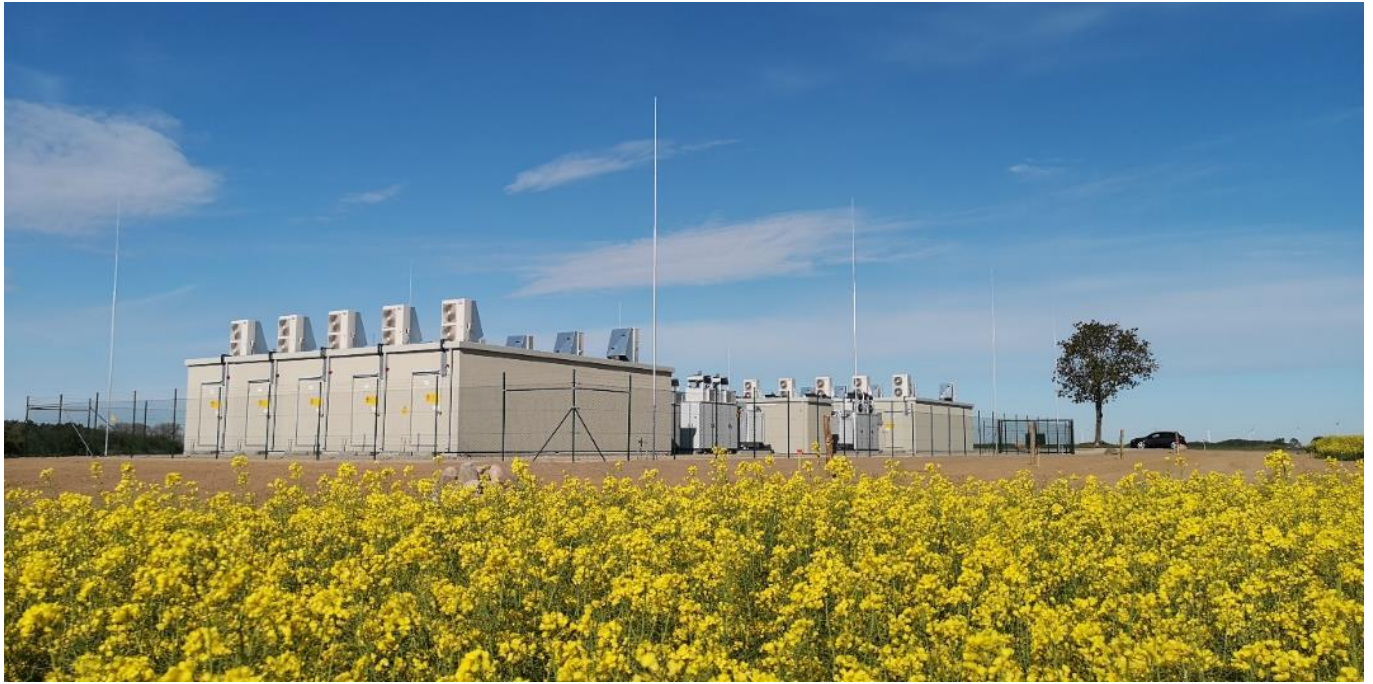
Figure 2.8: Li-Ion BESS implementation for a Renewable Energy facility (Source: Enel Green Power).
