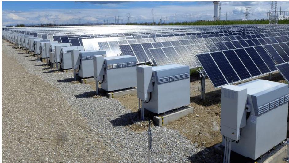
Figure 7.10 Example of battery storage units integrated as part of PV array (Source: nexttracker.com)
