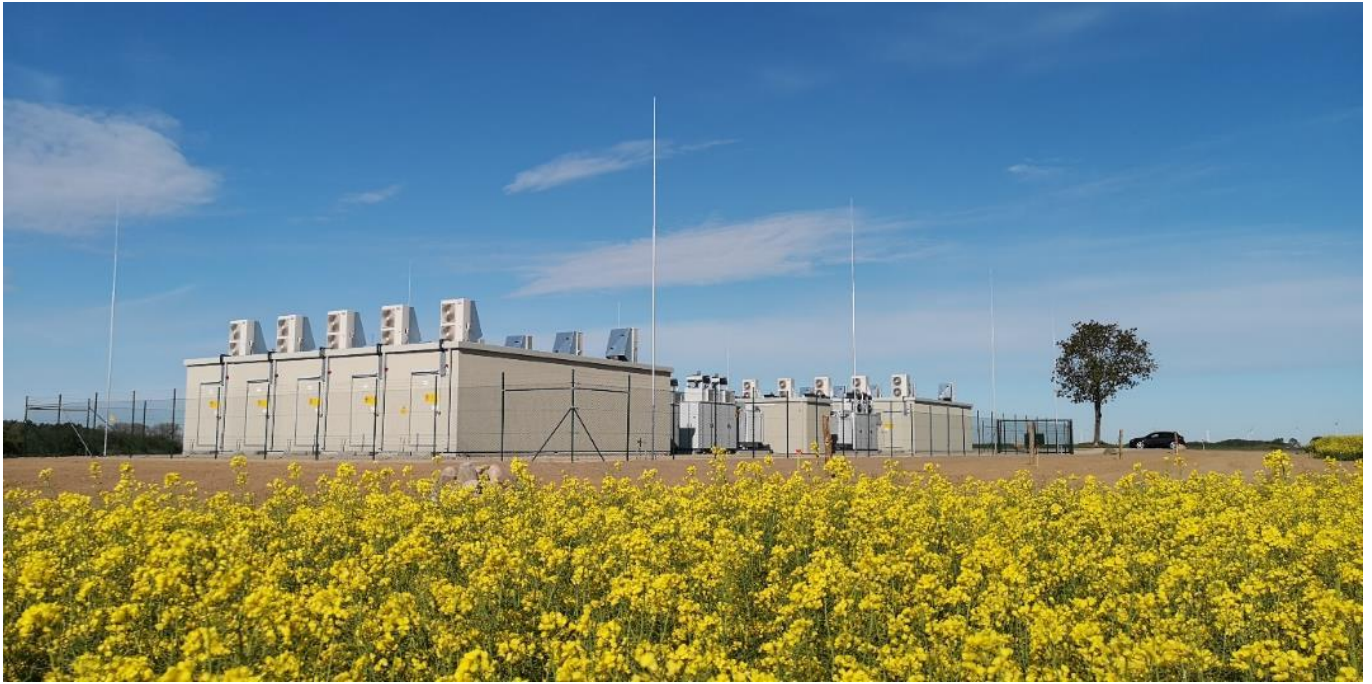
Figure 2.8: Li-Ion BESS implementation for a Renewable Energy facility (Source: Enel Green Power).
