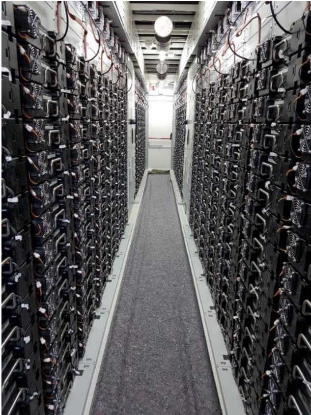
Figure 2.10: Li-Ion BESS internal design and implementation of a container used within a BESS. The image shows a series of sealed battery cell packs within a containerised module (Source: Enel Green Power).
