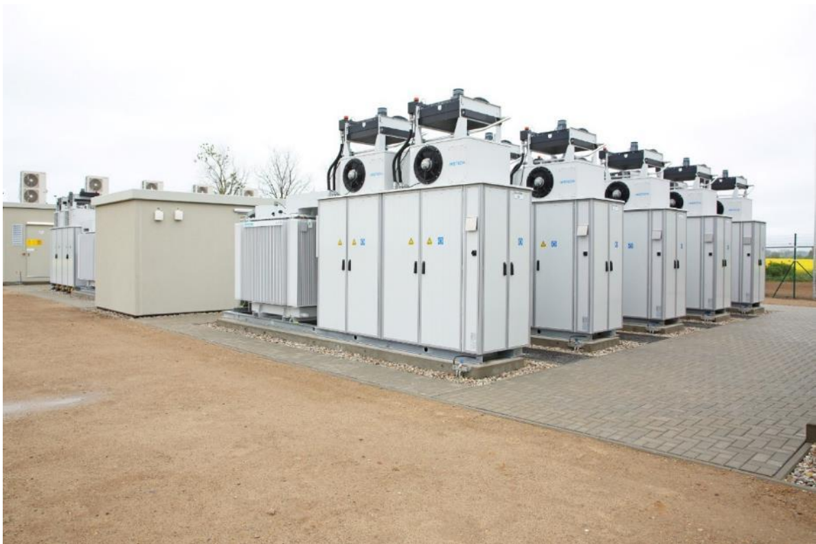
Figure 2.9: Li-Ion BESS containerised modules located within the BESS enclosure footprint (Source: Enel Green Power).
