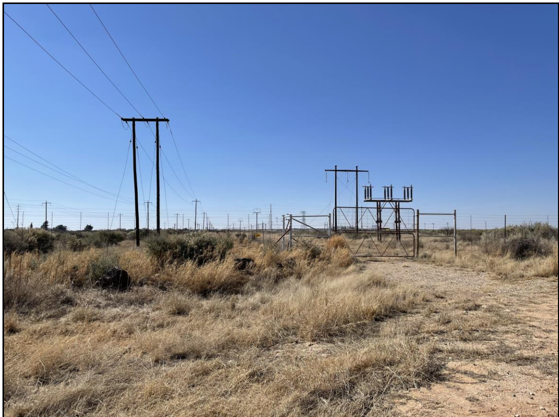
Figure 8: The Bophirima Substation and existing power line infrastructure at the proposed Woodhouse 1 Substation (Alternative B1) site.
