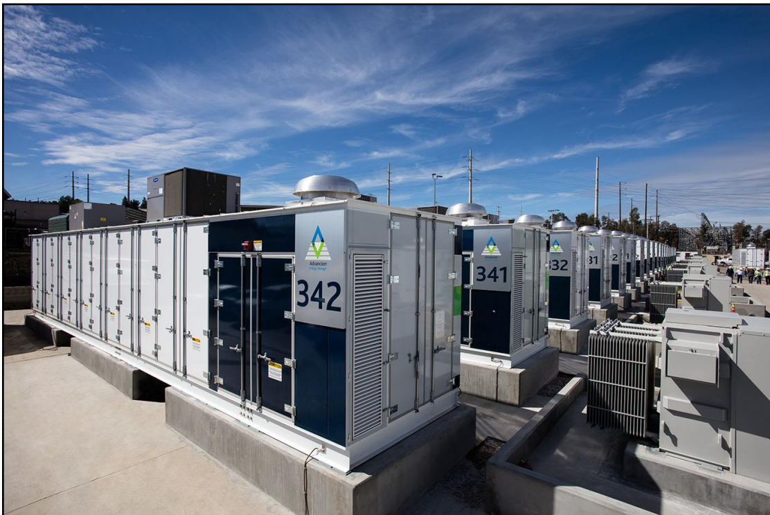
Figure 4: Close up view of a BESS facility (Photo: Greenbiz.com).
