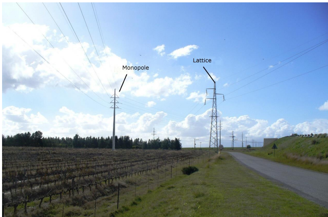
Figure 6: Typical 132 kV power line structures
