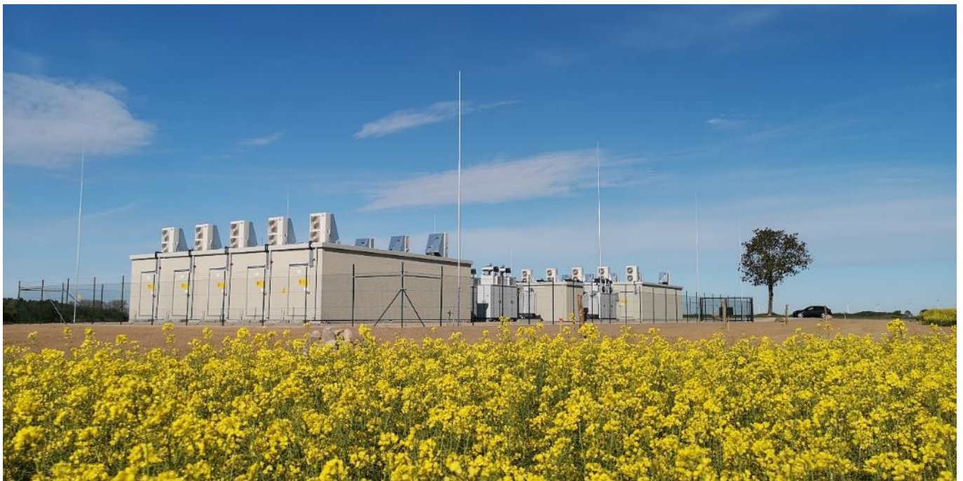
Figure 2.9: Li-Ion BESS implementation for a Renewable Energy facility (Source: Enel Green Power).
