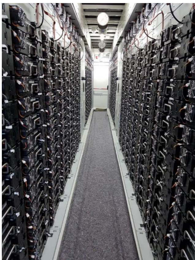
Figure 2.11: Li-Ion BESS internal design and implementation of a container used within a BESS. The image shows a series of sealed battery cell packs within a containerised module (Source: Enel Green Power).
