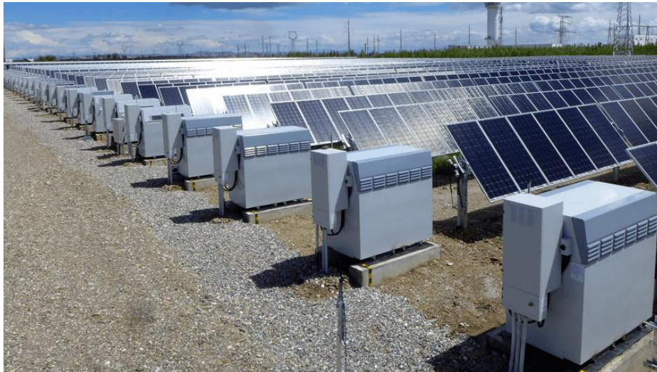
Figure 7.11 Example of battery storage units integrated as part of PV array (Source: nexttracker.com)
