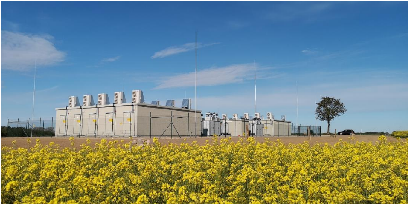
Figure 2.9: Li-Ion BESS implementation for a Renewable Energy facility (Source: Enel Green Power).
