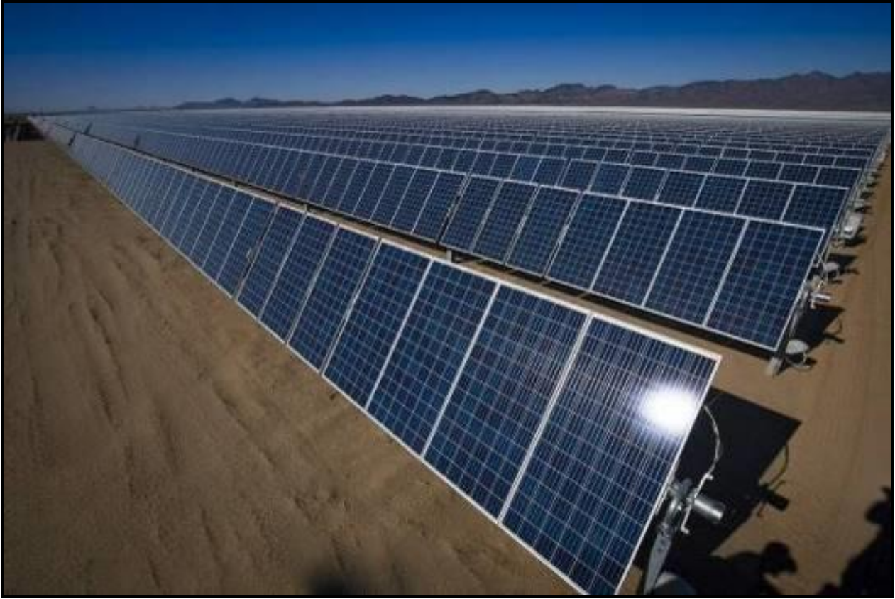
Photograph 1.1: Typical PV SEF facility
