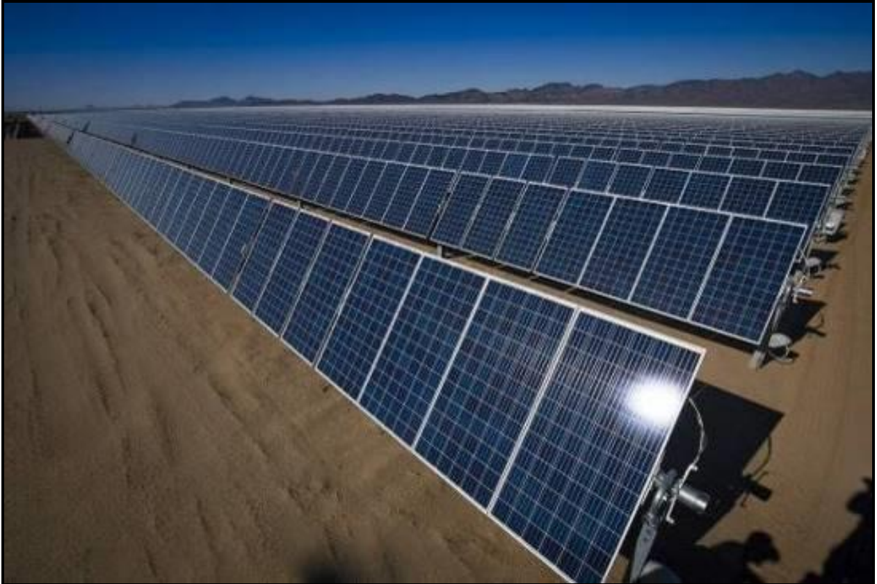
Photograph 1.1: Typical PV SEF facility
