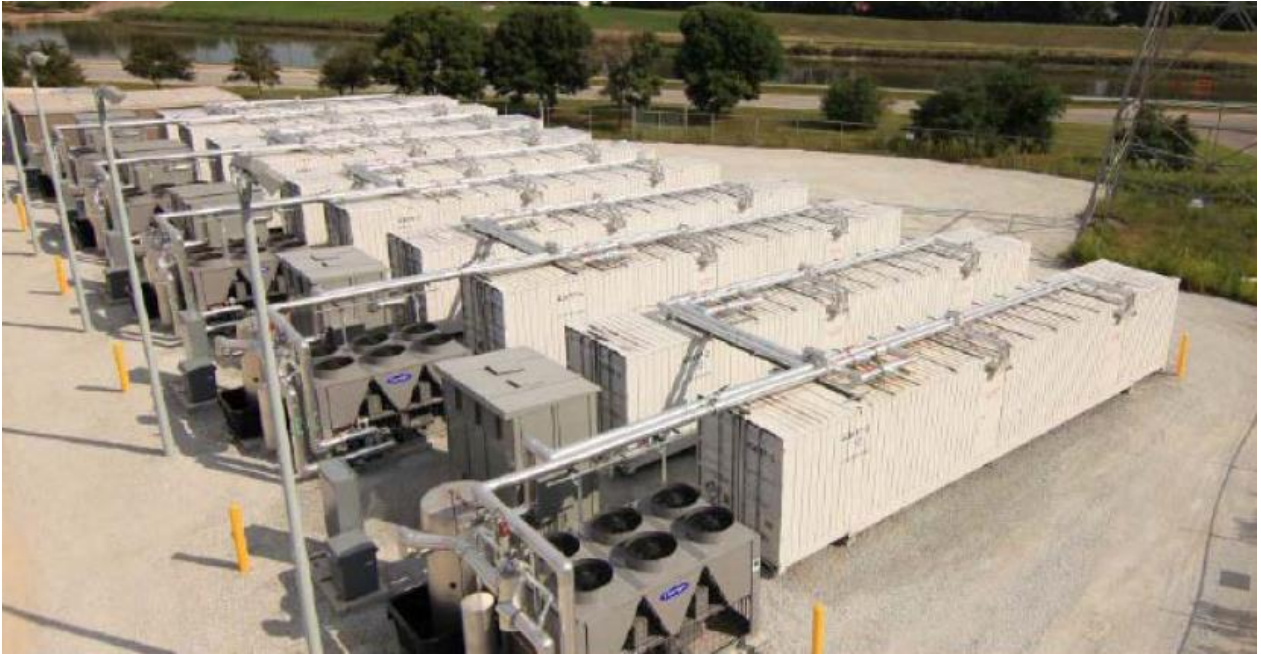
Figure 1.2: Example of Battery Energy Storage System (BESS)
