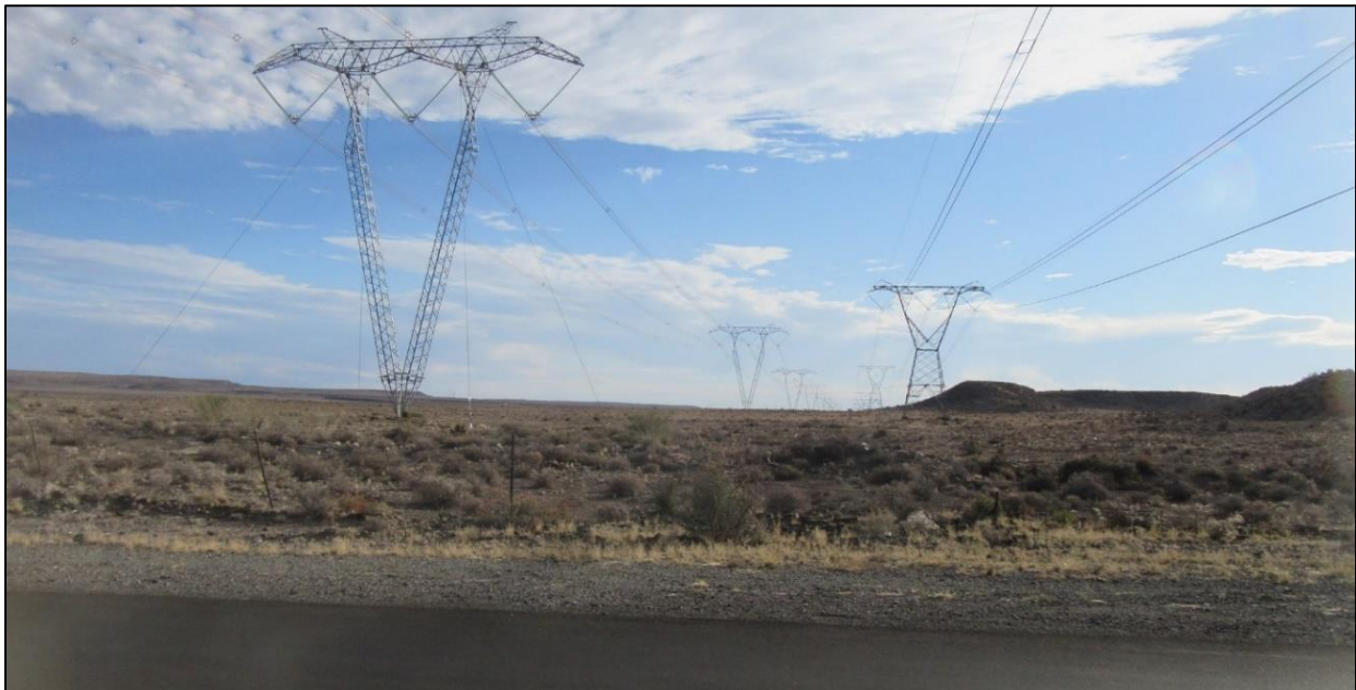
Photograph 3.6: Existing 2 x 400 kV line corridor traversing the R61 approximately 5.6 km south-east of Beaufort West
