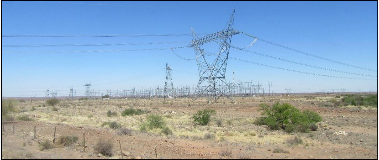
Photograph 3.4: Eskom’s Droeërivier MTS, seen from the north from along the N12
