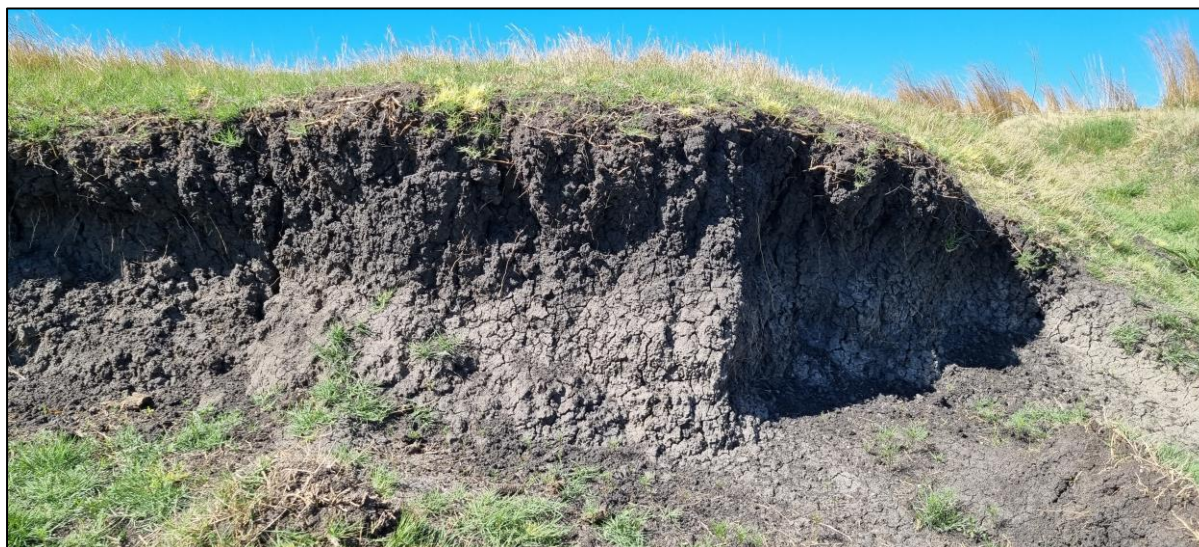
Figure 6-17 Example of erosion within HGM 1
