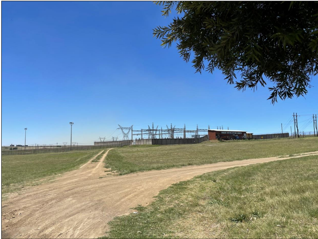
Figure 5: The Goedehoop Substation at the Riaan Rademan Training Facility.
