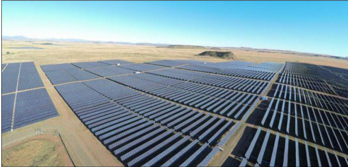
Figure 3: Aerial view of PV arrays. (Photo: Scatec Solar South Africa).
