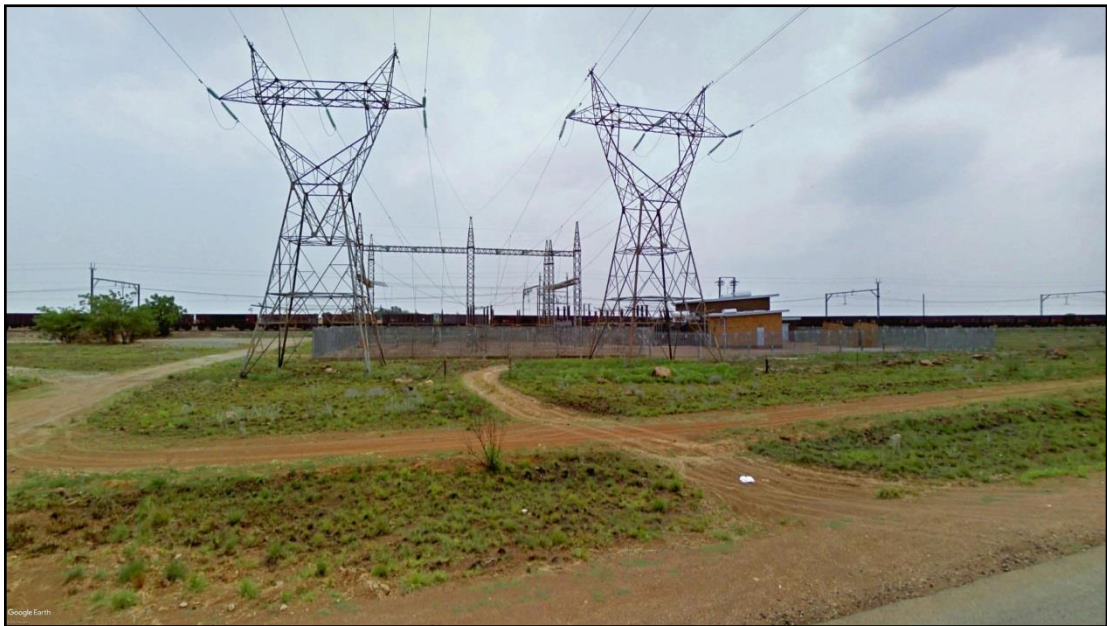
Figure 5: The Dean Traction 132kV Substation.
