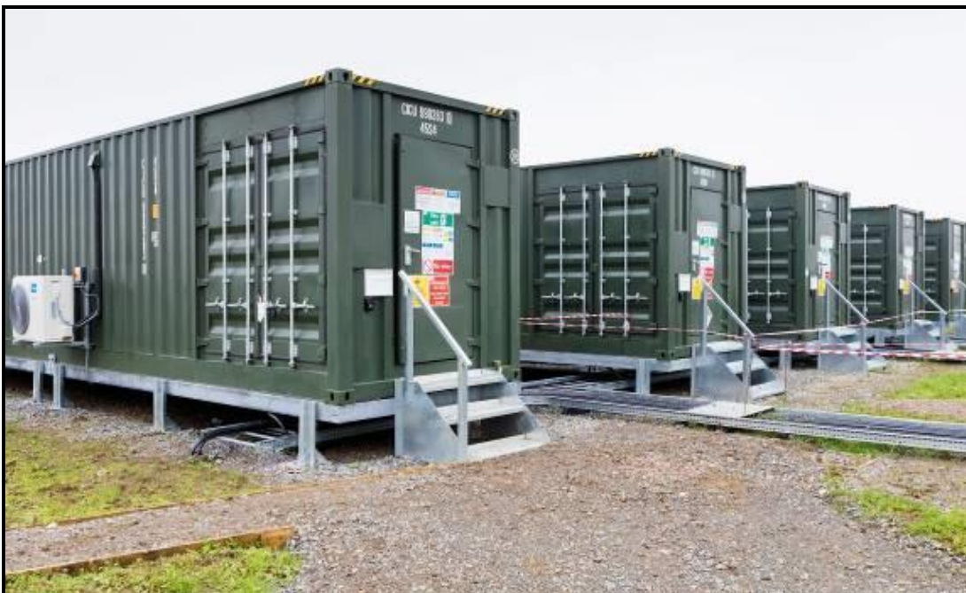
Photograph 1.2: Example of BESS located in storage containers
