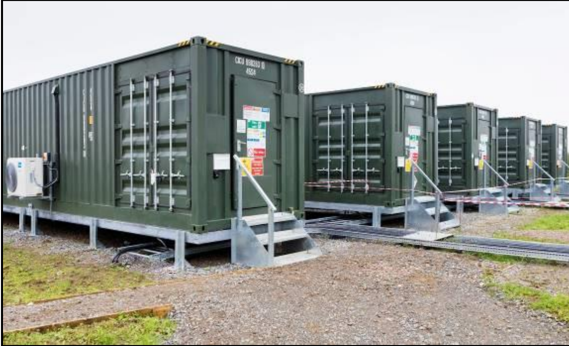
Photograph 1.2: Example of BESS located in storage containers
