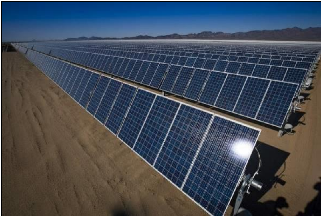
Photograph 1.1: Typical PV SEF facility
