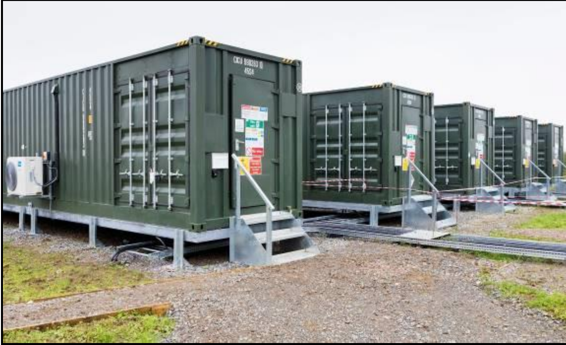
Photograph 1.2: Example of BESS located in storage containers
