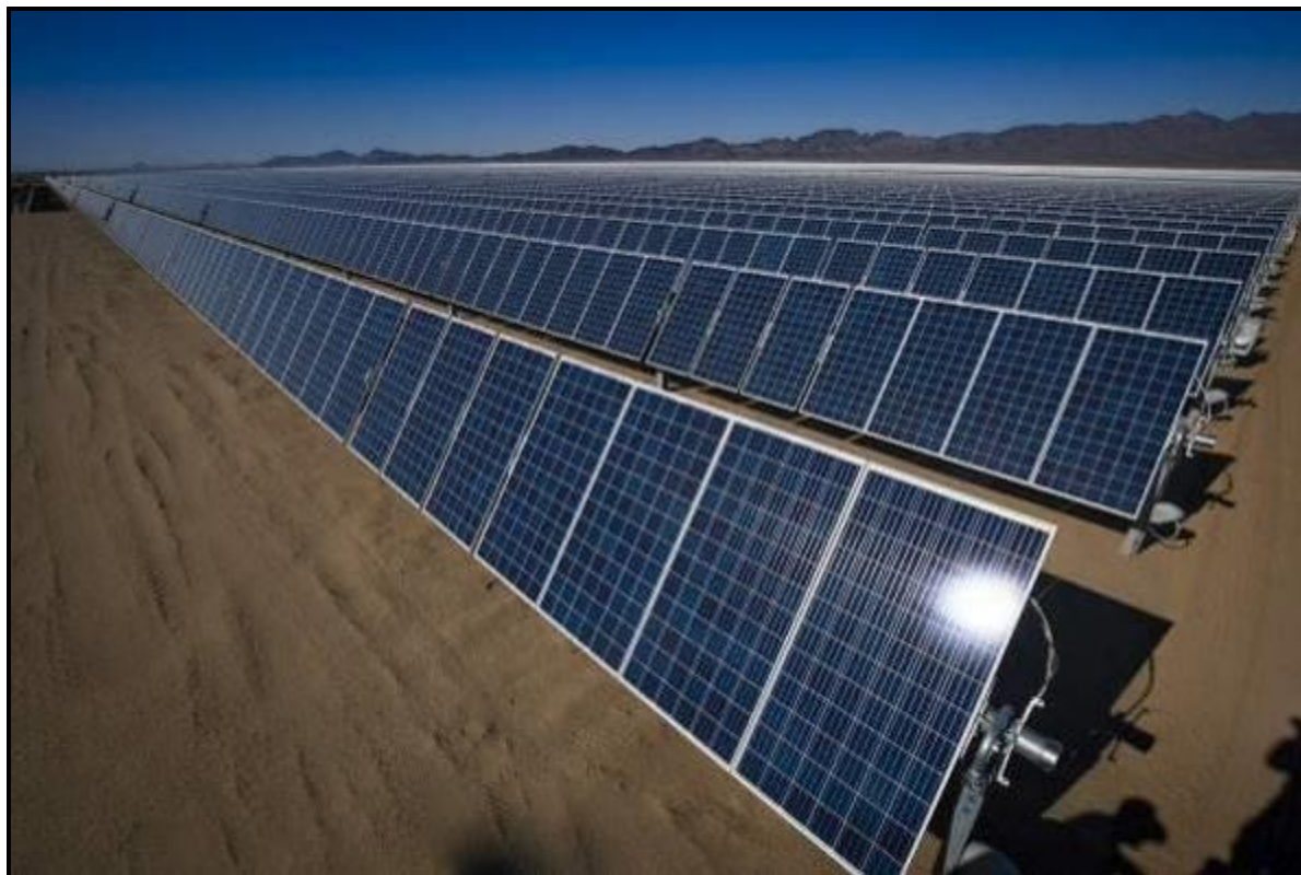
Photograph 1.1: Typical PV SEF facility
