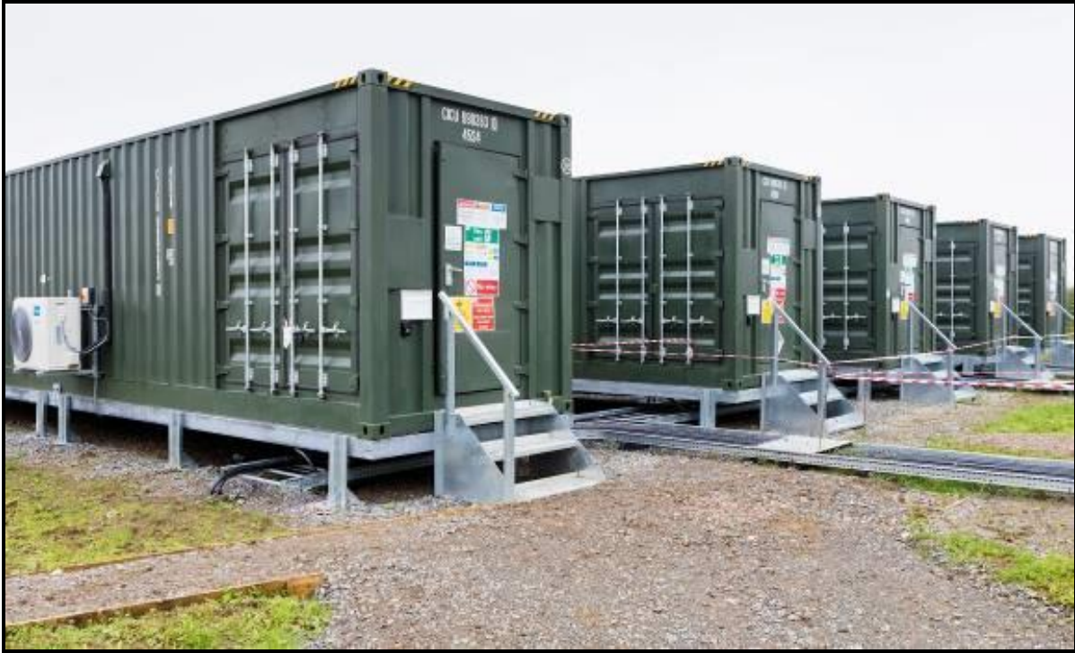
Photograph 1.2: Example of BESS located in storage containers
