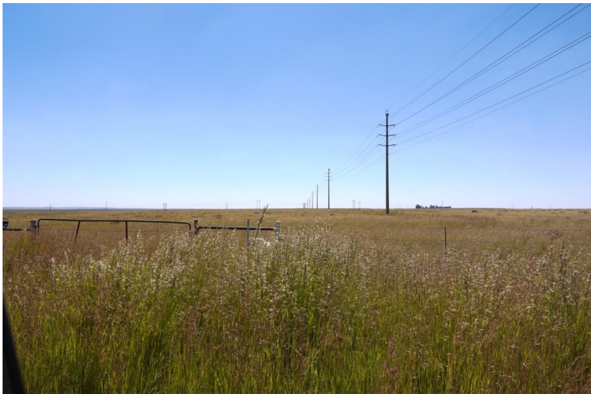
Plate 10 - A view along the line of a 132kV overhead power line with monopole towers
