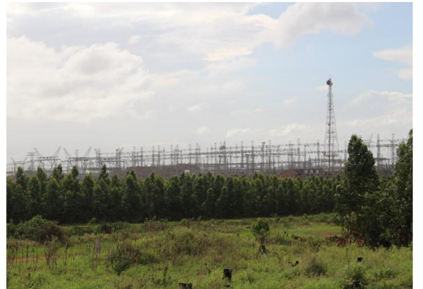
Plate 18 - Sub-station & Communication Tower
