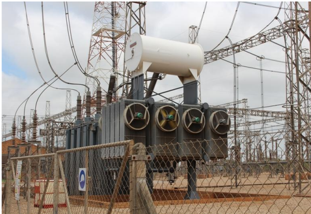
Plate 17 - Transformer showing oil reservoir and fans for cooling
