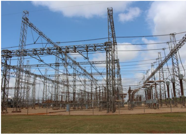
Plate 15 - Sub-station Bus Bars maximum height 22.5m
