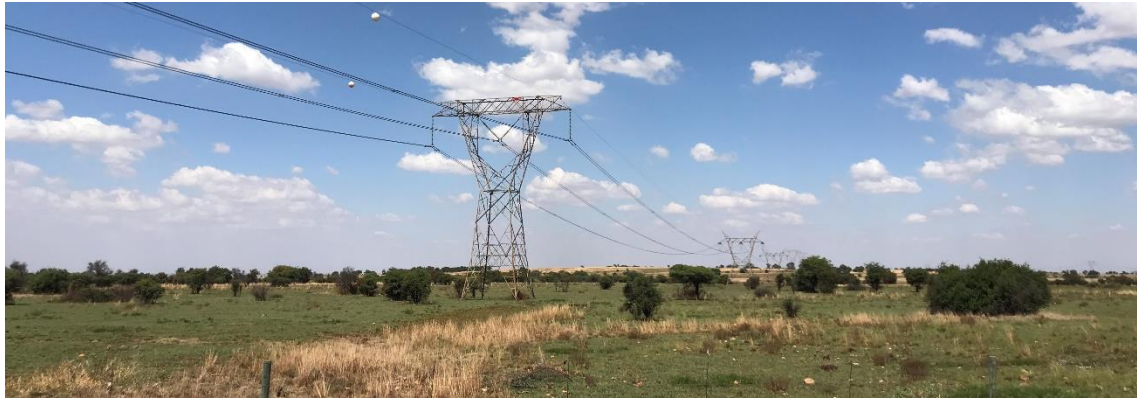
Figure 6: Existing power lines in the study area
