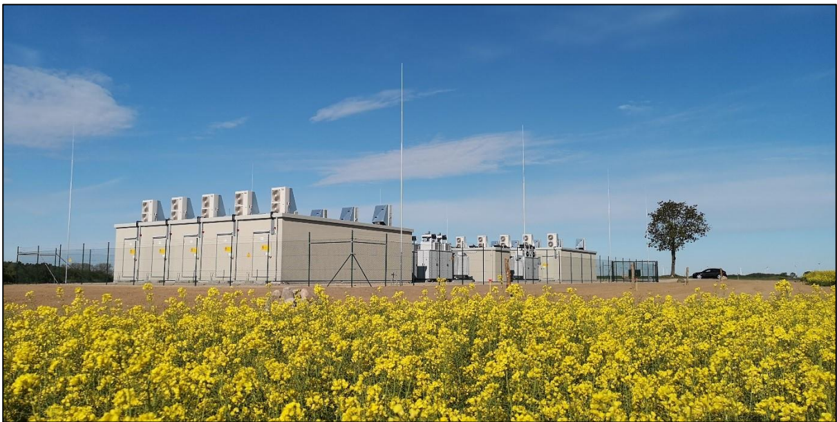
Figure 2.2: Li-Ion BESS implementation for a Renewable Energy facility (Source: Enel Green Power).
