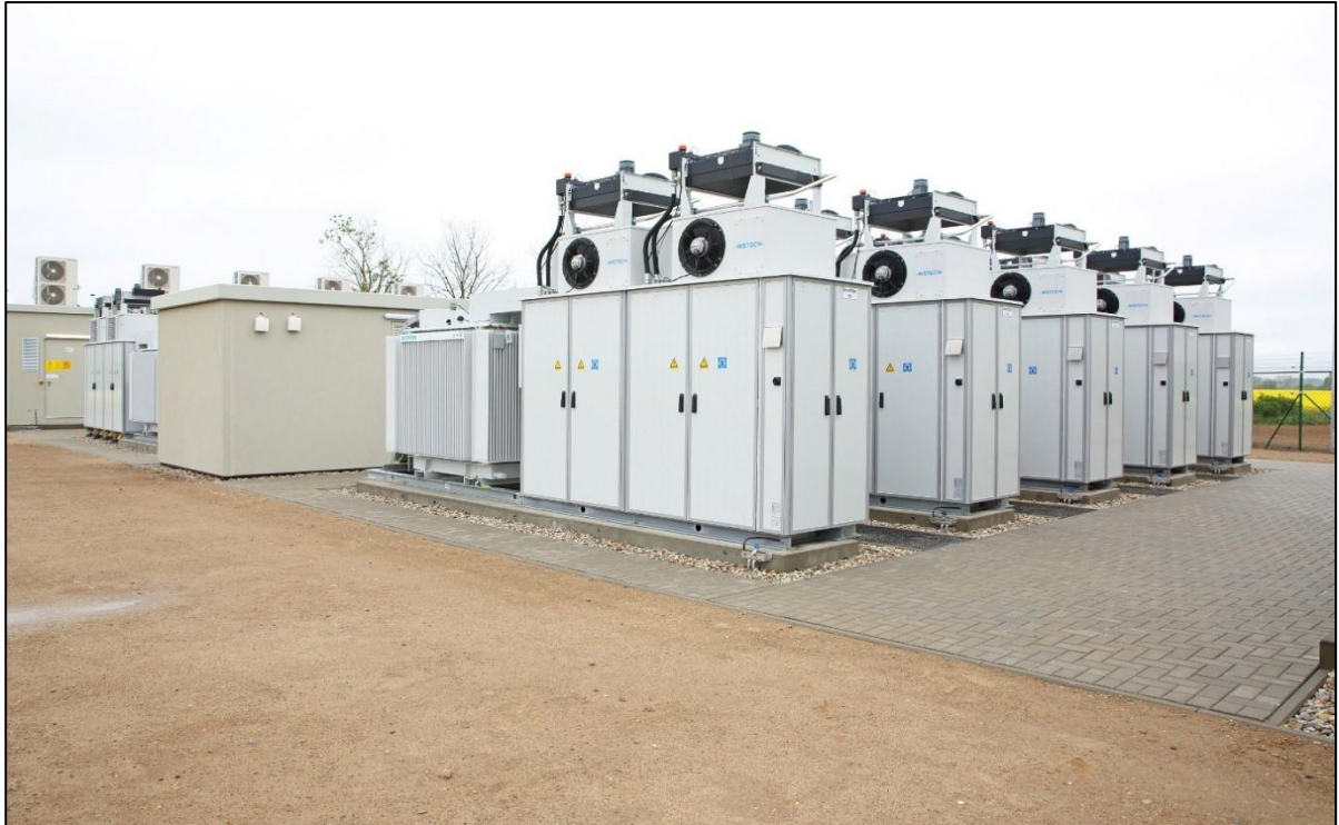
Figure 2.3: Li-Ion BESS containerised modules located within the BESS enclosure footprint (Source: Enel Green Power).
