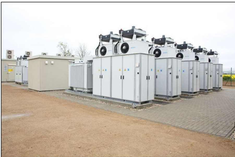
Figure 2: Li-Ion Bess containerised modules located within the BESS enclosure footprint (Source: Enel Green Power)
