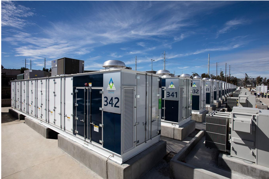
Figure 5: Close-up view of a BESS facility (Photo: Greenbiz.com).
