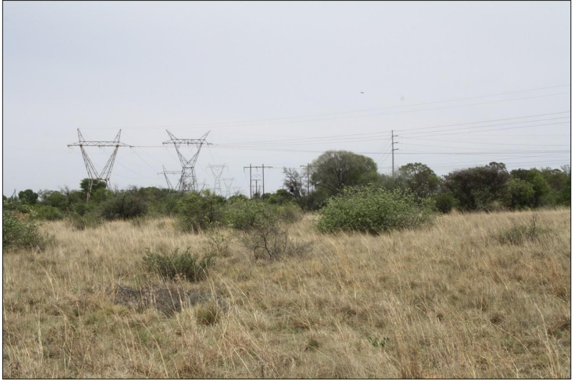
Figure 8: Power lines near the Watershed Substation.
